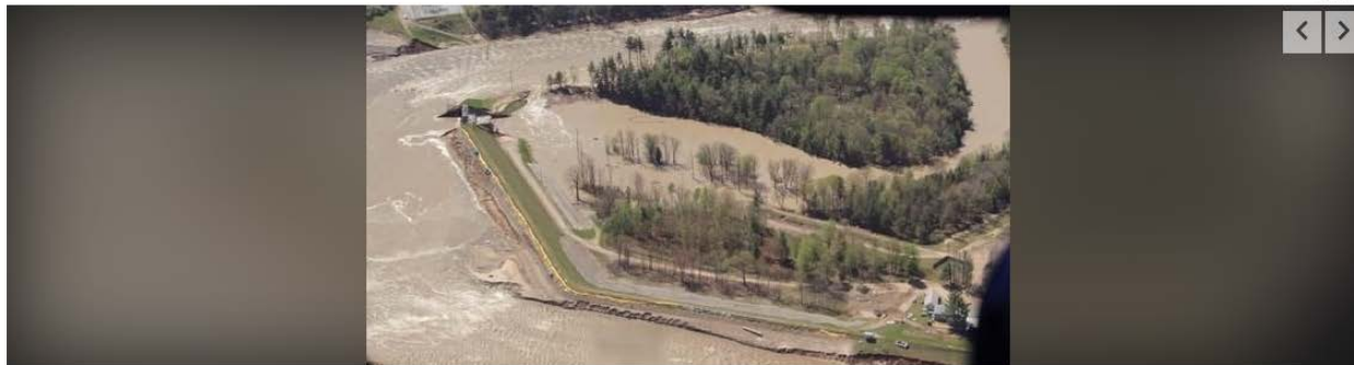
The Edenville Dam failed on May 19, 2020.
