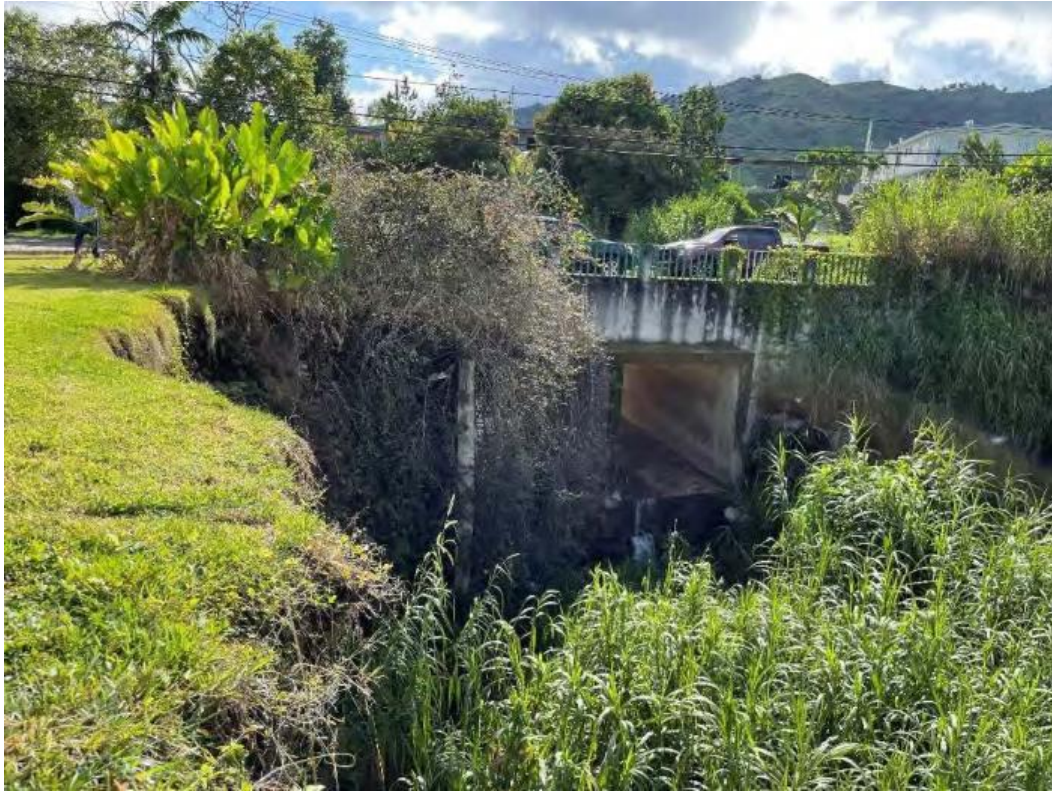
Top to bottom: Extensive right bank erosion and potential collapse risk of home and gazebo. Erosion along the bridge wingwall and the right bank. Photo Credit: Jaca & Sierra, Geotechnical Engineers – Puerto Rico
