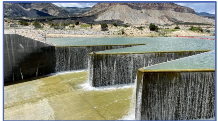
The auxiliary spillway at the Millsite Dam shown here on, June 20, 2023 shows a complete reconfiguration of the auxiliary spillway.
