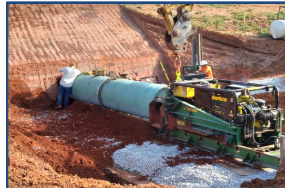
A new concrete pipe was installed using a "jack and bore" technique.
