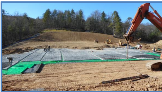
The control and outlet sections of the auxiliary spillway were covered with articulated concrete blocks to prevent surface erosion. The spillway was then covered with soil and seeded to hide the concrete blocks.
