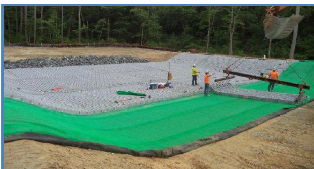
The earthen auxiliary spillway was armored with articulated concrete blocks which were then covered with soil and seeded to grass to hide the concrete.
