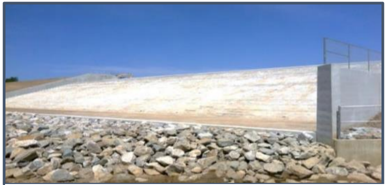
The dam was rehabilitated in 2013 to add a 300-foot wide roller compacted concrete spillway
