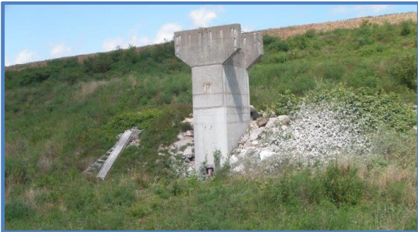
Three feet of the top of the concrete principal spillway tower was cut off to lower the spillway inlet.
